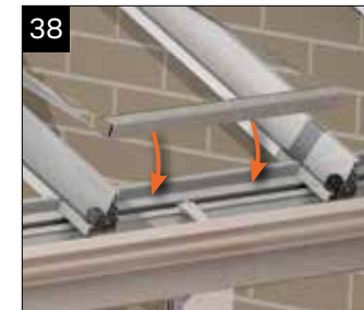
At this point the roof should be glazed. Any ridge support may be removed. Insert the glazing between the rafters ensuring that it is centralised.
