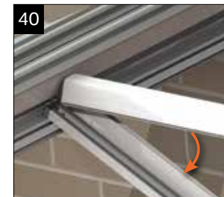
Once the roof has been fully glazed and glazing stops secured, work your way around the roof fitting the glazing bar top caps. These should be angled in at the ridge first before forcing the top cap down along the bar length. Ensure to fully engage w grip clip.
