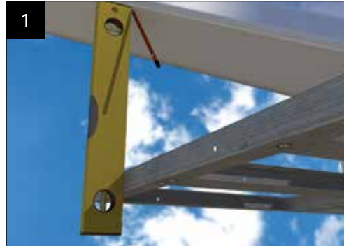
1 Using a level, plumb up off the horizontal frame and mark the outer bottom edge of the valley cladding on both sides (Mark "A")
