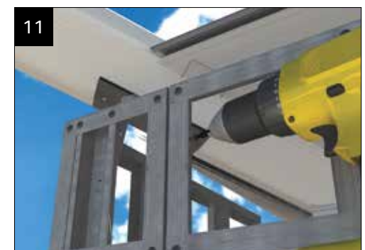
11 Fit the vertical frames. Fix the frames into the valley corner infill and the horizontal frames.
