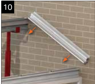
Continue to support the ridge and offer up the starter bars at the host wall. Locate on to the single bolts at the ridge and eaves.
