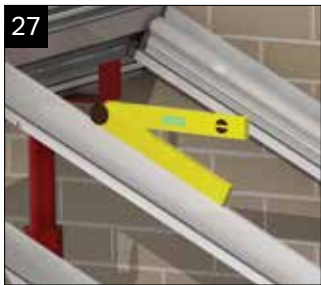
Check that the pitch of the roof is correct. Your Surveyor should have provided a drawing/a copy of the roof confirmation which displays the pitch.
