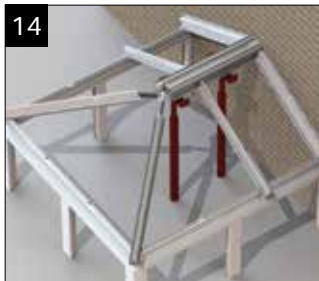
Using the location plan, repeat these steps until all rafters that meet the ridge have been fitted in the correct position and have been secured.
