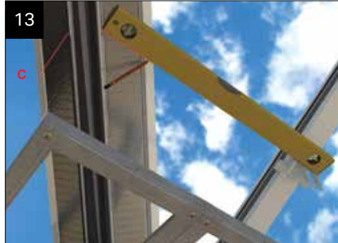
13 Using the bracket positions, level through and mark off the valley marked 'C'.
