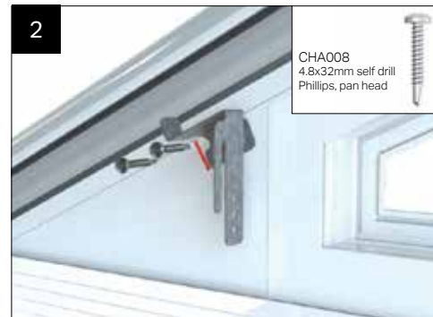
Take the gable bracket (CHA019R right hand shown). The back edge of the bracket should butt up to the pencil line. Align the top face of the gable bracket with underside of starter bar cladding.
