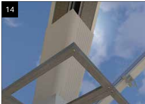
14 Measure and fit the standard valley undercladding NVU-V between the eaves and mark 'C'. Scribe to suit.
