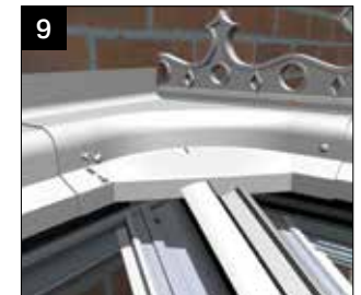
9 The joint between the full and half ridge PVC top caps is sealed by the use of a capping connector. This needs to be trimmed to suit. Bed the capping on suitable silicone and fix using the plastic rivets provided.
