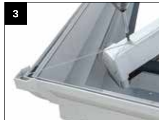
3 Finally secure the corner by screw fixing the wire tie to the glazing bar using self drilling screw CRN010
