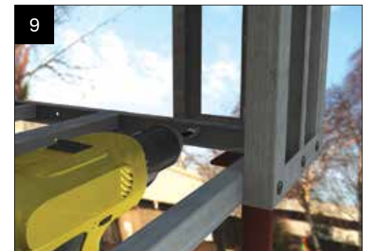
9 Fit the valley corner infill panel to the horizontal frame, level up and secure to the valley plate.
