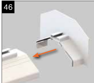
46 Now fit the ridge flashing trim to the ridge top cap, apply a bead of silicone inside to secure.
