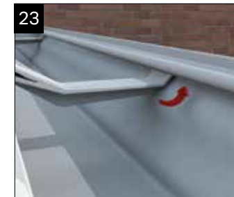
Clip the front of the bracket into the lip on the gutter. PVCu components like the gutter are easier to manipulate when warm. In cold conditions more 'force' may be required.
