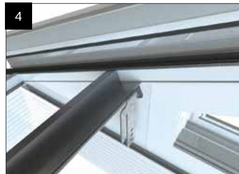
Offer into position the cloaking panel support trim - the nose of the closure trim must be notched back as shown (at the gable side only).
