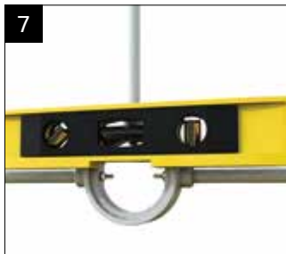
Now, finally check that the horizontal elements are level and the vertical element is plumb. CHECK THAT THE SIDE FRAMES ARE STILL PLUMB. Spanner tighten the boss nyloc nuts.
