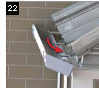
Locate the back edge of each section of gutter into the slot in the gutter bracket.
