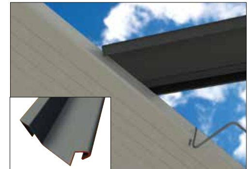
In valley situations the closure trim sits onto the valley drip profile. The nose of the closure trim must be notched as shown above, this allows the trim to sit flat.
